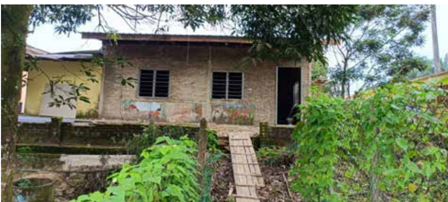
(Top) Before EnQuest's intervention, one of the classroom buildings was in disrepair. (Bottom) Now, the building is in the midst of being refurbished with new walls, tiles, lighting, and roof.
