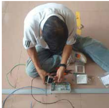
Setting up the computer lab with new wiring, IT equipment, air conditioning, and other electrical appliances.
