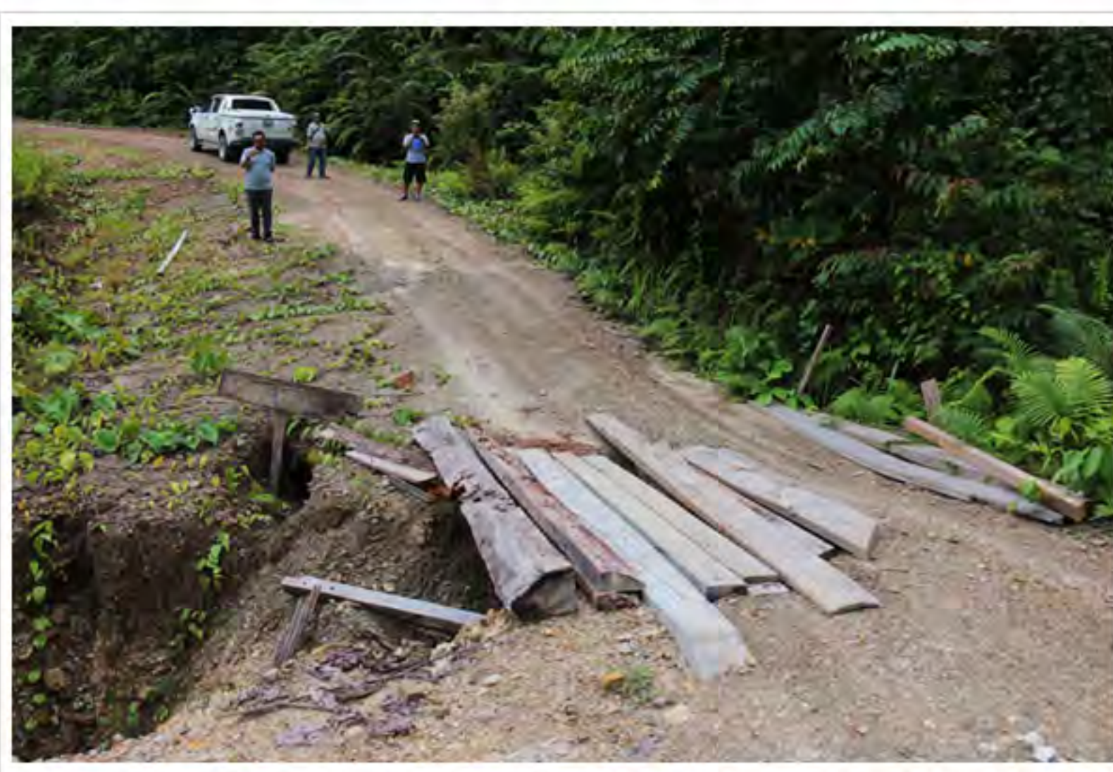
This damaged section of the off-track road has yet to be repaired.
